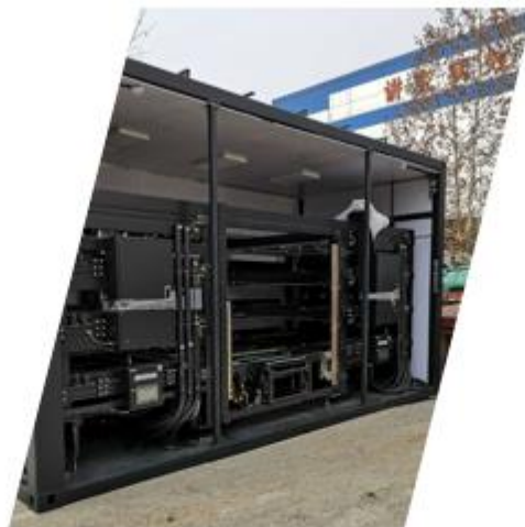
新能源换电站 New Energy Charging Station
